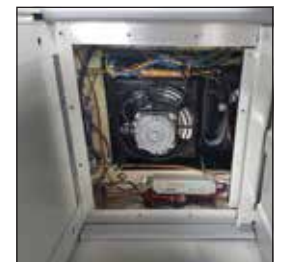
A5. Condenser compartment
